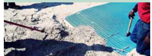
FIG. 3 - COVER ENDS WITH SAND TO PREVENT TRIPPING
